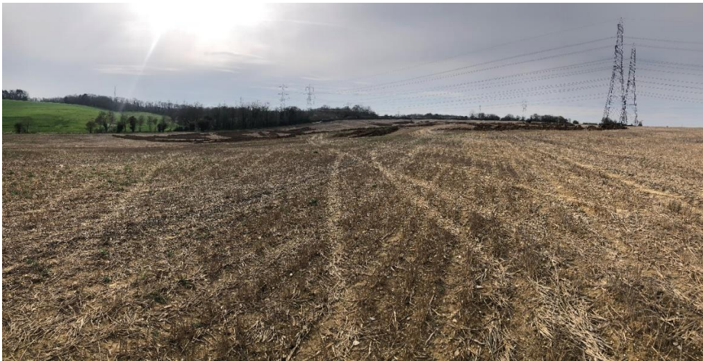
Figure 1 – Progress West of the EA cables and South of the Gas lines
